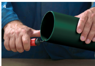
4 Remove the sharp edges on the inside
